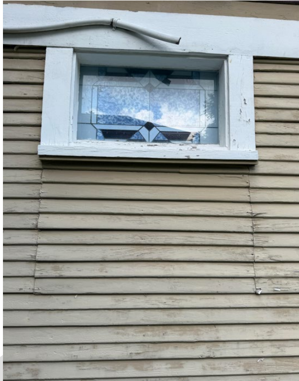
Figure 1-The existing window opening shows ghosting that indicates the original window's size and configuration, meaning the outline of the historic frame is still visible and the current unit does not match the original dimensions.
